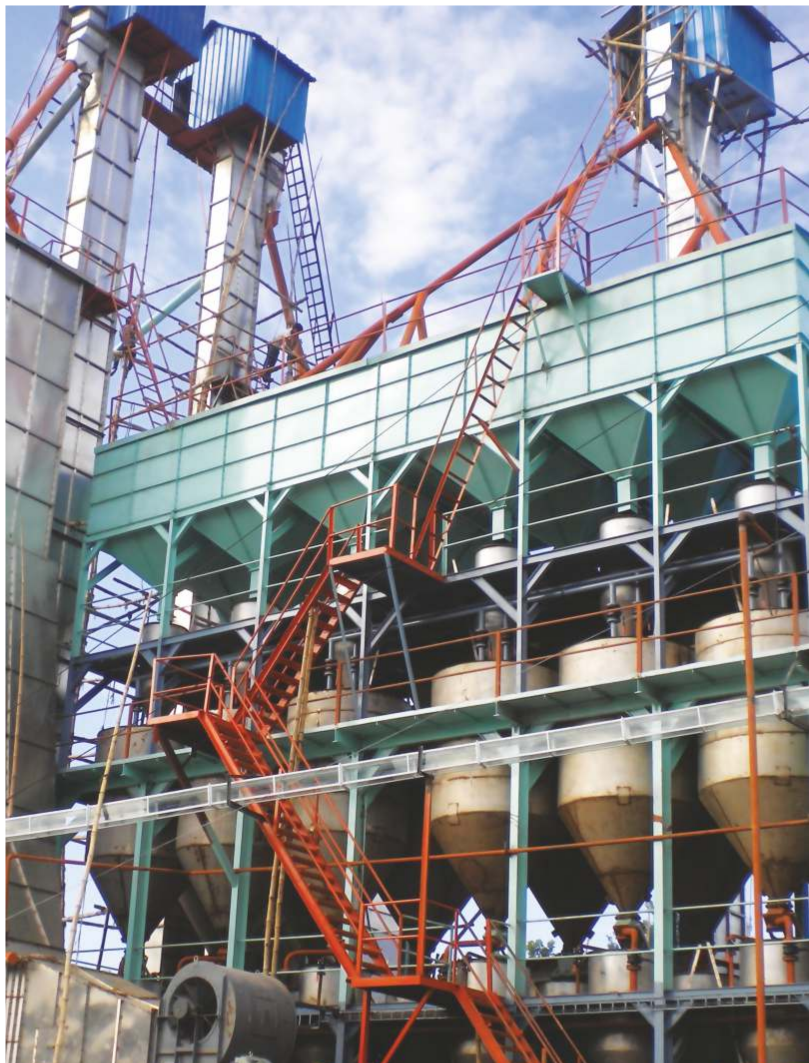
2 X 24 TON THREE STAGE PLANT
