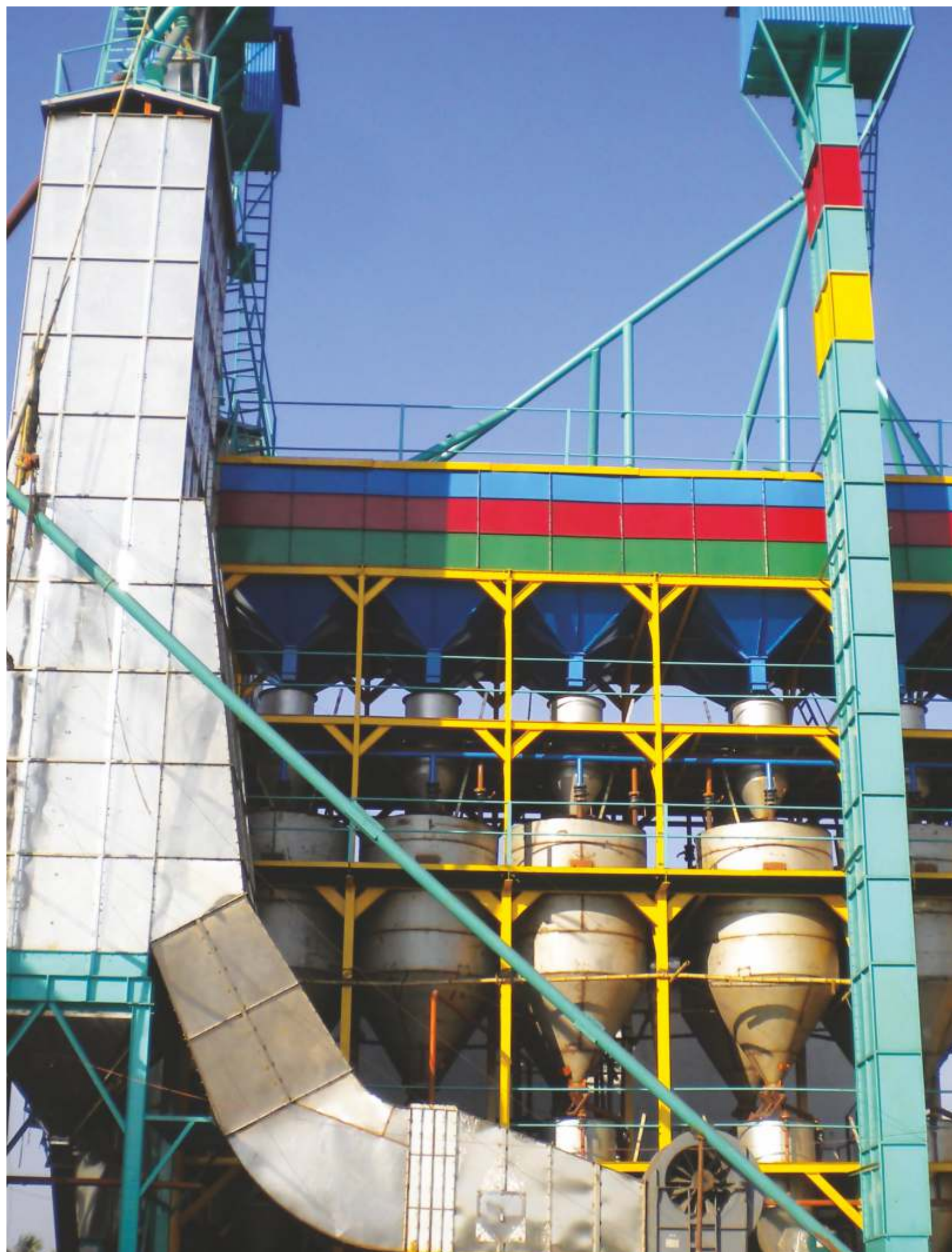
2 X 24 TON THREE STAGE PLANT
